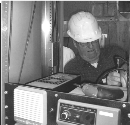
Howard emptying the old rack cabinet.
