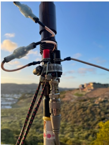
Figure 2. The new 20 meter antenna is mounted in a similar manner to the railing.
