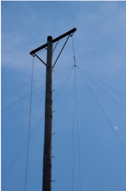
The lead is pulled up, with 8 top load radials hanging on it
