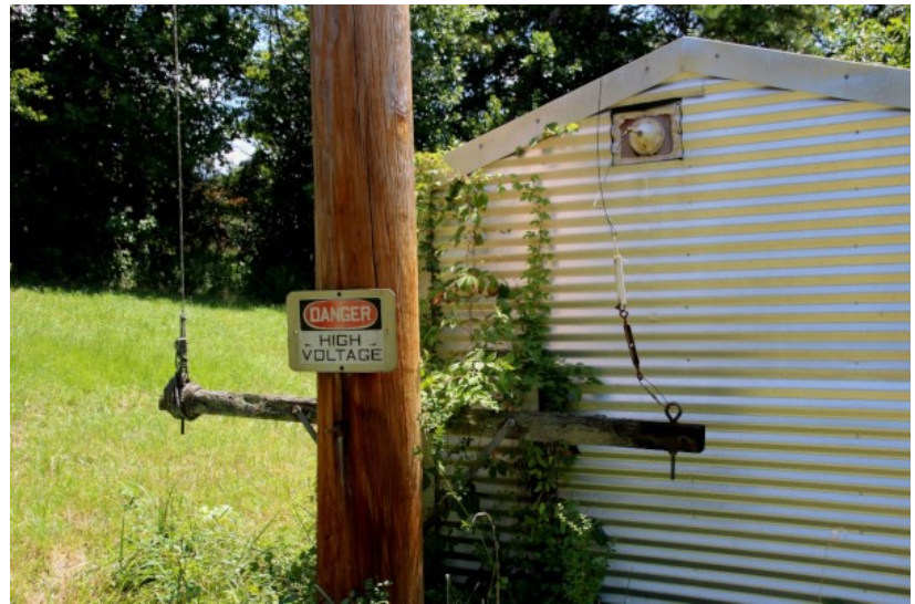
From the transmitter shed, the lead goes up to the top of the pole, and then down again to the bottom to adjust tension
